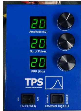
Photo of TPS external controller located in engine control room
